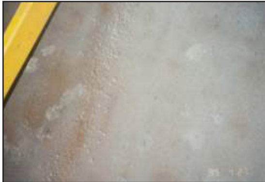
Corrosion and pitting on the spillway gate
